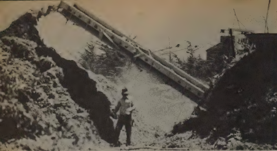
▲ The hammermill assembly in the tub grinder is feeding shredded material onto the conveyor.
